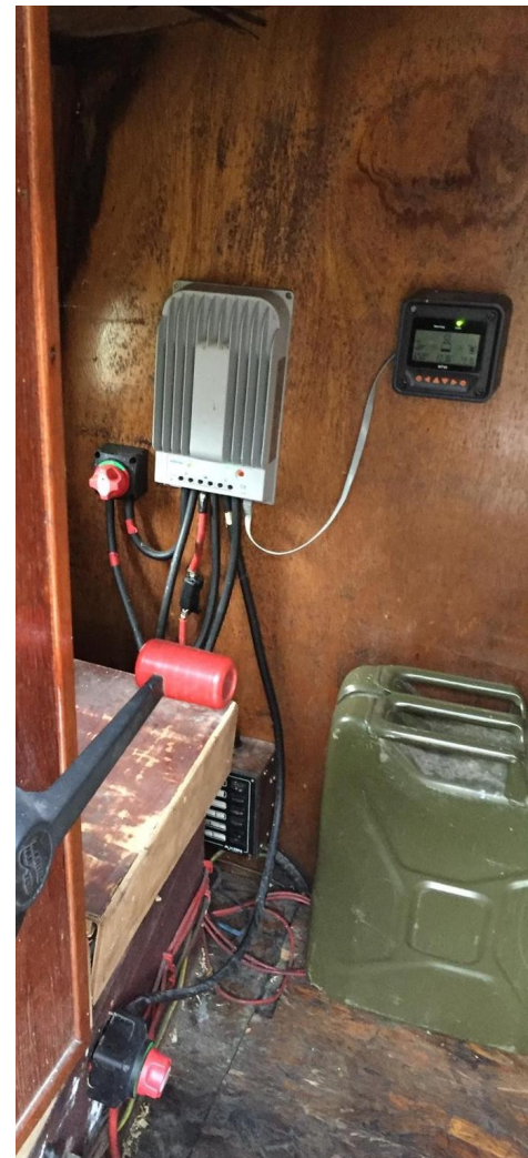
Solar charge regulator and monitor
